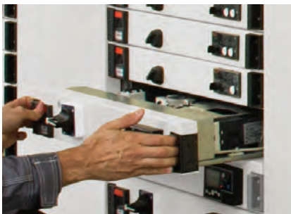
Fig. E32: Distribution switchboard with withdrawable functional units in drawers
