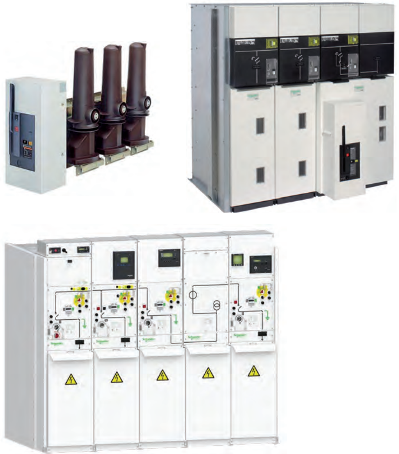
Fig. B25: Schneider Electric SM6 and Premset switchboards including MV/LV transformer protection with circuit breaker associated to self-powered relay
