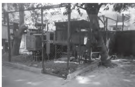
Fig. B59: Outdoor substation without enclosure
